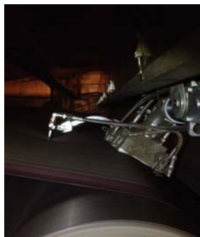
View of M-clean cleaning system in operation
