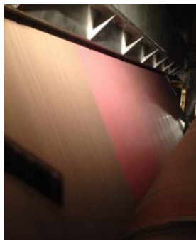
View of Unirun dryer felt during cleaning cycle
